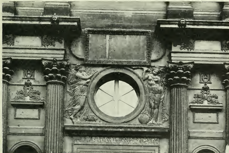
DETAIL OF FAÇADE OF LESCOT AND GOUJON: - LOUVRE. CALLED PAVILION HENRI II.
